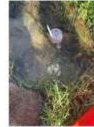
Seeing the size and scope of leaks like this one helps our operators determine the best course of action.
